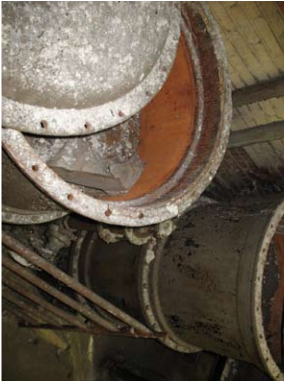
Figure 6 Decommissioned tanks connected to potable water supply
