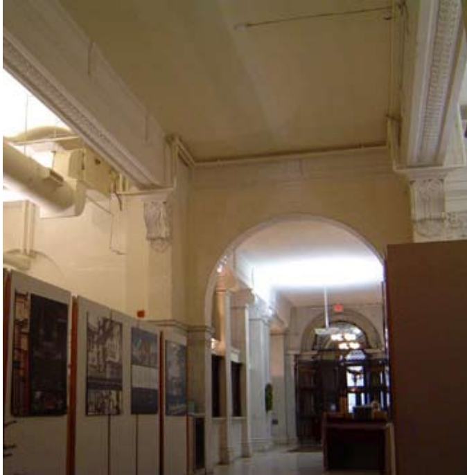
Figure 3 In the existing historic area, the cement open structure with plaster architectural details limited the amount of pipes passing through open areas.
