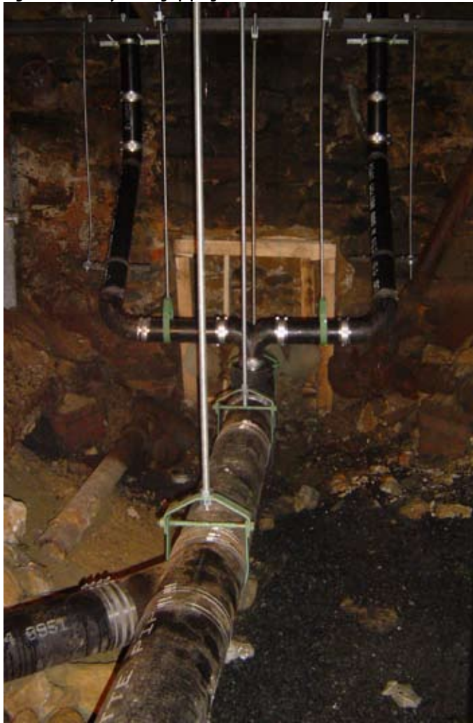
Figure 6 Sanitary drainage piping
