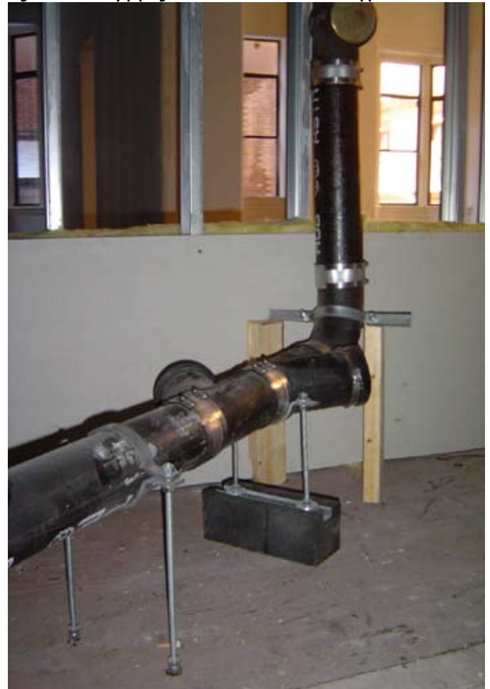
Figure 4 Sanitary piping installed below a raised floor application
